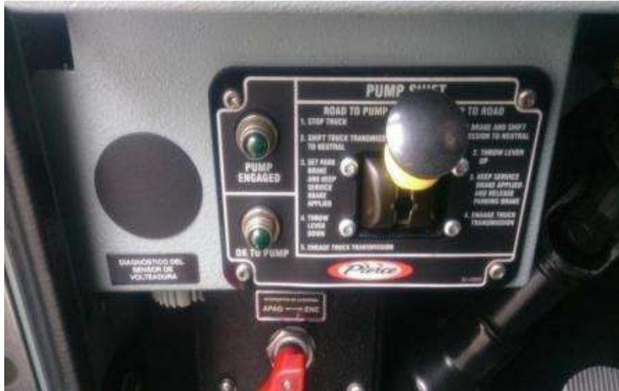
Figura 7. Pump Power Shift MA-03
